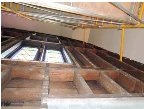
Bowed wall, with discontinuous studs.
